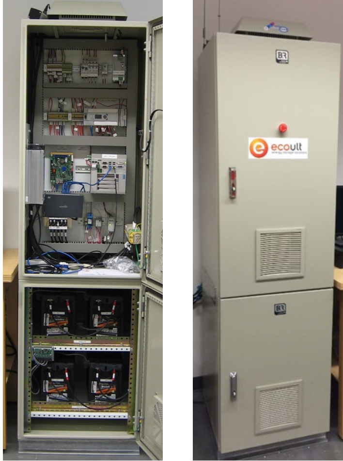
Figure 4. Battery cabinet and control/monitoring electronics enclosure.
